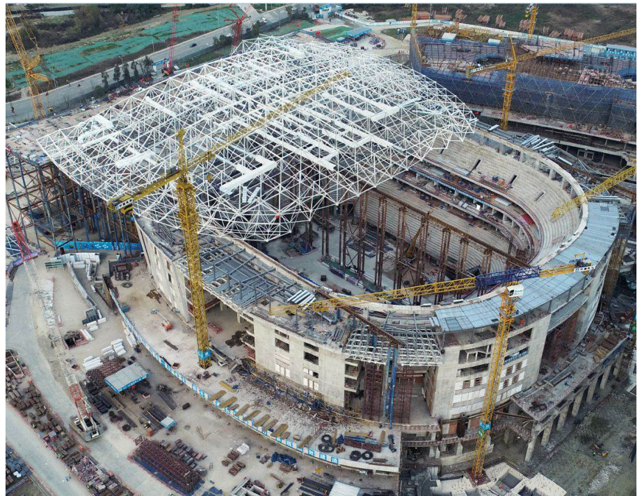
Left: Intelligent models are used to guide assembly on-site. Right: An image of the construction happening on-site. Courtesy of China Construction Eighth Engineering Division Corp. Ltd.
