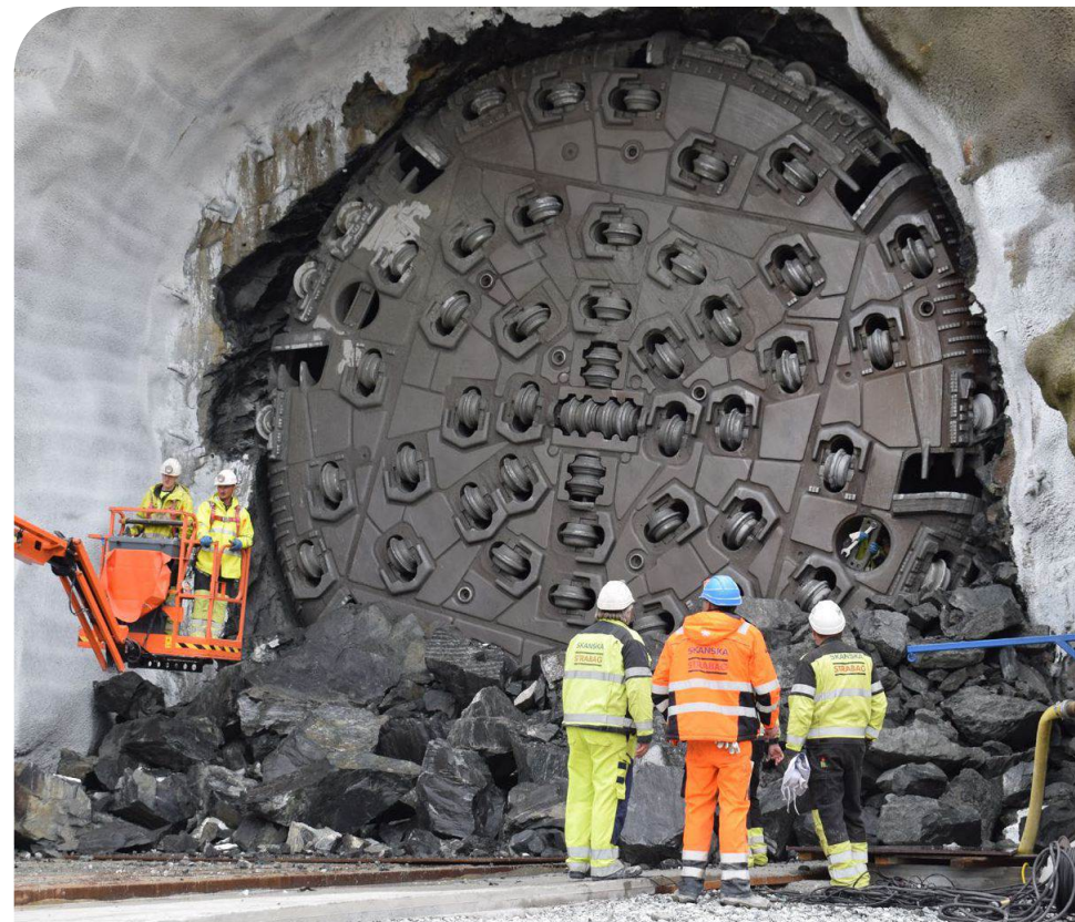
The tunnel-boring machine breaks through Ulriken Mountain in Bergen on Aug. 29, 2017. Courtesy of Warren Eversley/Bane NOR/Norconsult AS.
