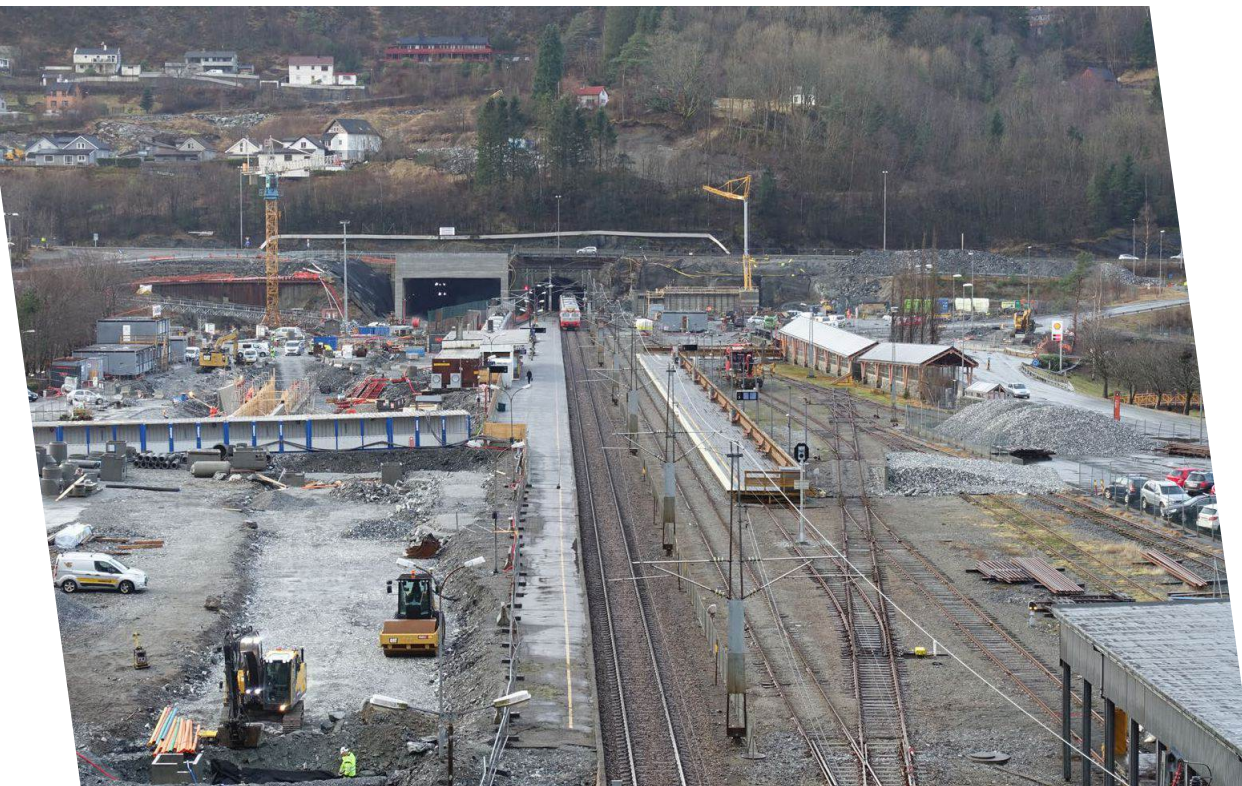
The Arna Station upgrade under construction, with a train coming from the existing tunnel and the new tunnel to the left. Courtesy of Ingvild Eikeland/Bane NOR/Norconsult AS.
